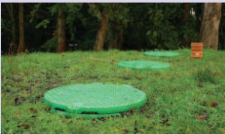
Underground tanks were installed to minimise visual impact, the underground tanks allow the ground above to be landscaped
