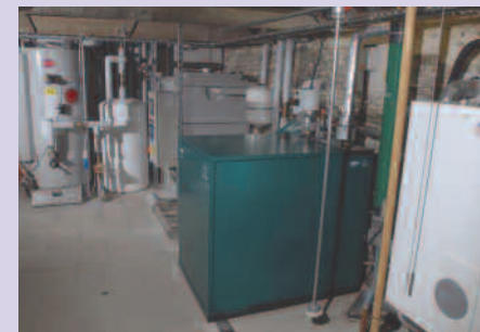
An LPG powered CHP unit can deliver in excess of 75 per cent fuel efficiencies
